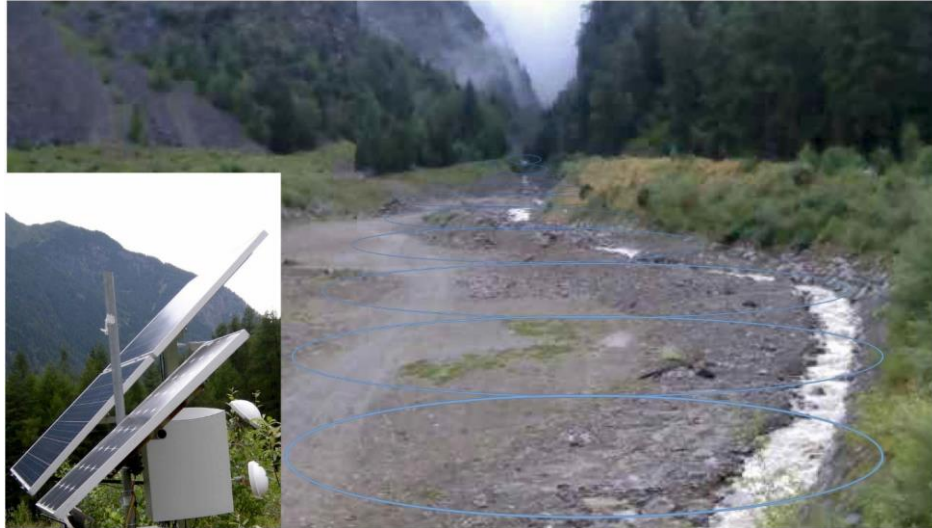
Installed RADAR-System (smaller picture) with 2 antennas and solar power supply in Umhausen/Tirol Austria and view from the RADAR-system with monitored area subdivided in range gates.
